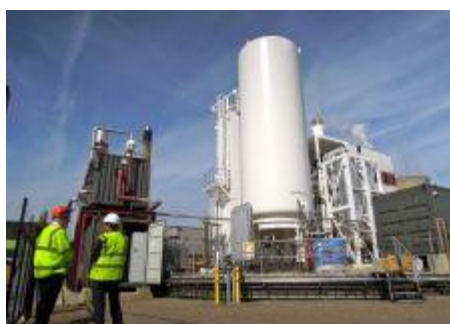
Fig 7. Linde Liquid Air Storage Tanks
